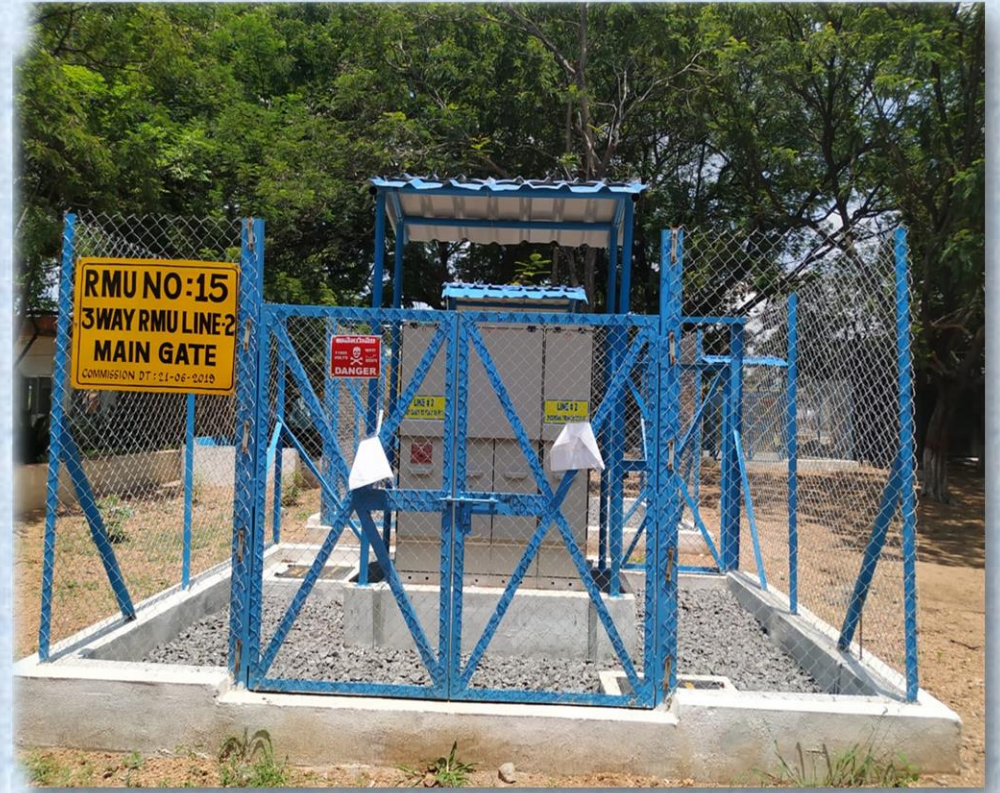
Commissioning of RMU under LT Package at Ramagundam completed in July 2019
